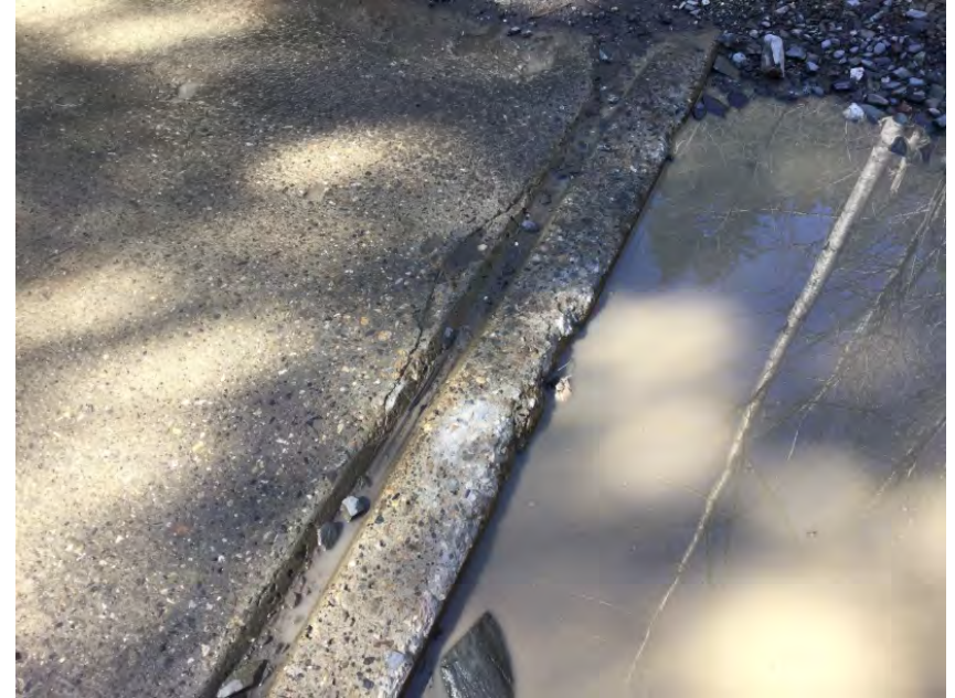
Damage to left approach panel and ballast wall
