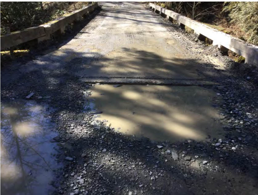
Potholes left approach
