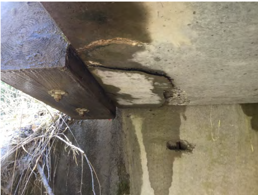
Damage noted to underside of panel 1 right approach
