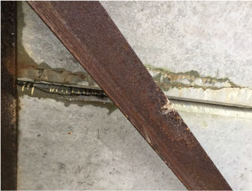
Damage noted to underside of panels
